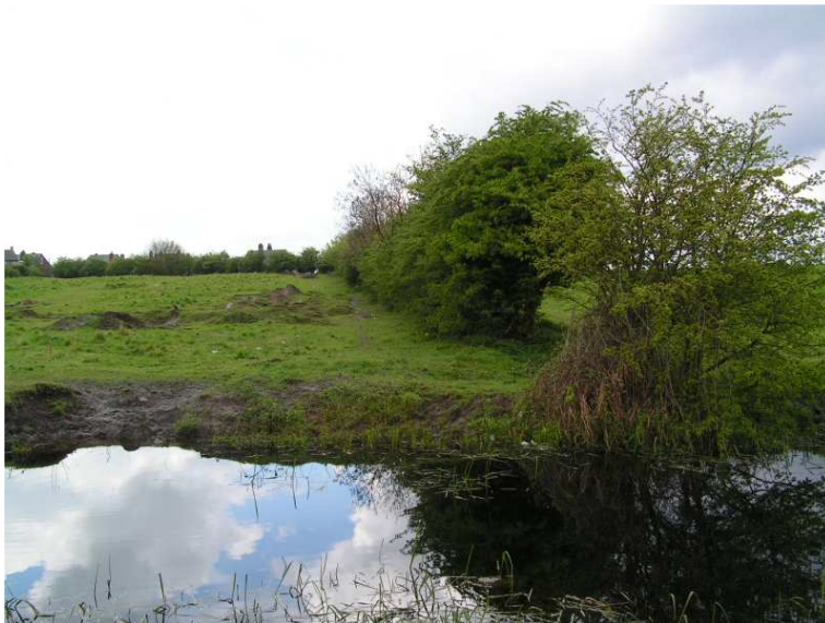
Off bank of canal at Norwood Bends showing erosion and subsidence.
